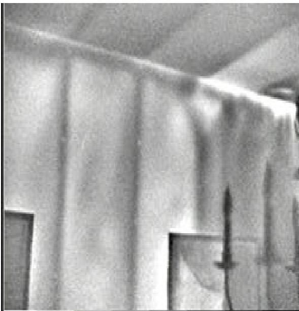
Infra-red image of Thermal Bridging
