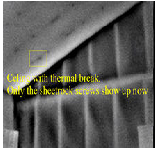
Infra-red image of Thermal Bridging
